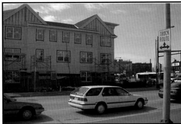
New elderly housing being constructed on University Ave. in northern Merriam Park
